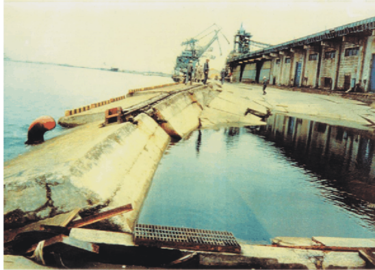
Figure 1.1 Damage to a quay wall at Akita Port. The seabed is liquefied after the 1983 Nihonkai–chubu earthquake (Sumer, 2014a).
